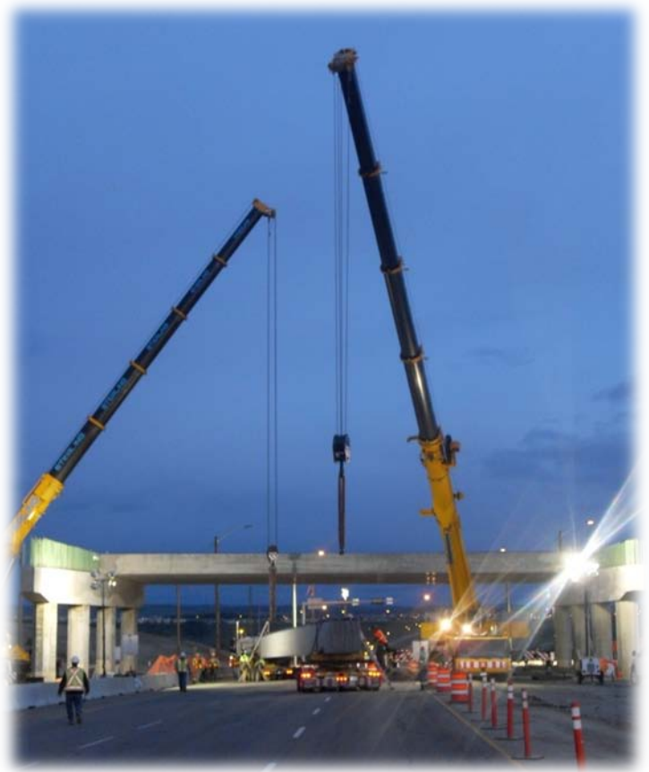
Bridge girder installation June 2011 at Highway 22X and the Cranston Blvd/McKenzie Lake Blvd SE interchange.
